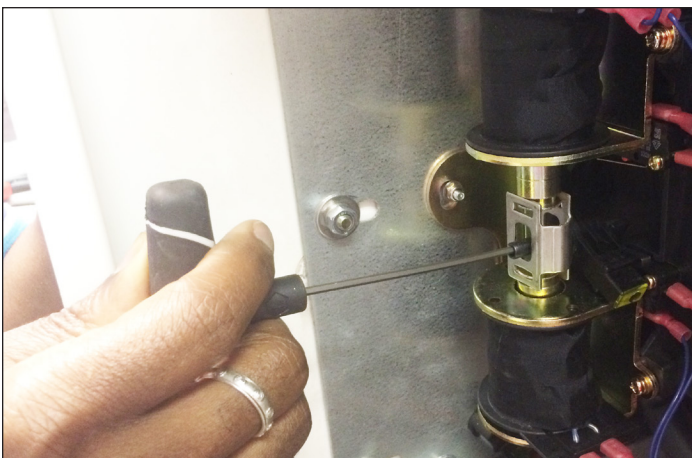
Fig. 19 Checking transfer switch movement
